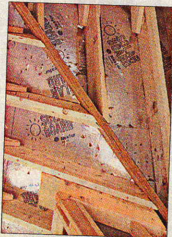
Ray says proper insulation installation is the first step in creating an energy-efficient home.
